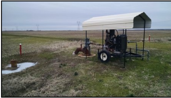
13 : Typical natural gas powered agricultural well located on the Subject Property
