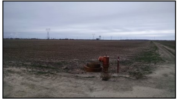
20 : Irrigation riser associated with the electric well on the Subject Property (facing southeast)
