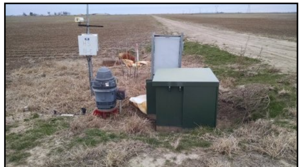
18 : Electric powered well (and associated ground-mounted transformer) in the north-central area of the Subject Property
