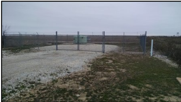
3 : Ground-mounted transformer located in the southwest corner of the Subject Property, possibly associated with the Denso facility
