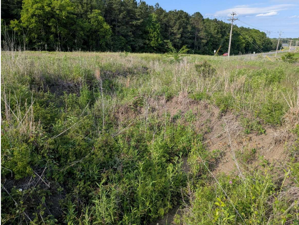
Photo 23: Erosive feature (north-central)
