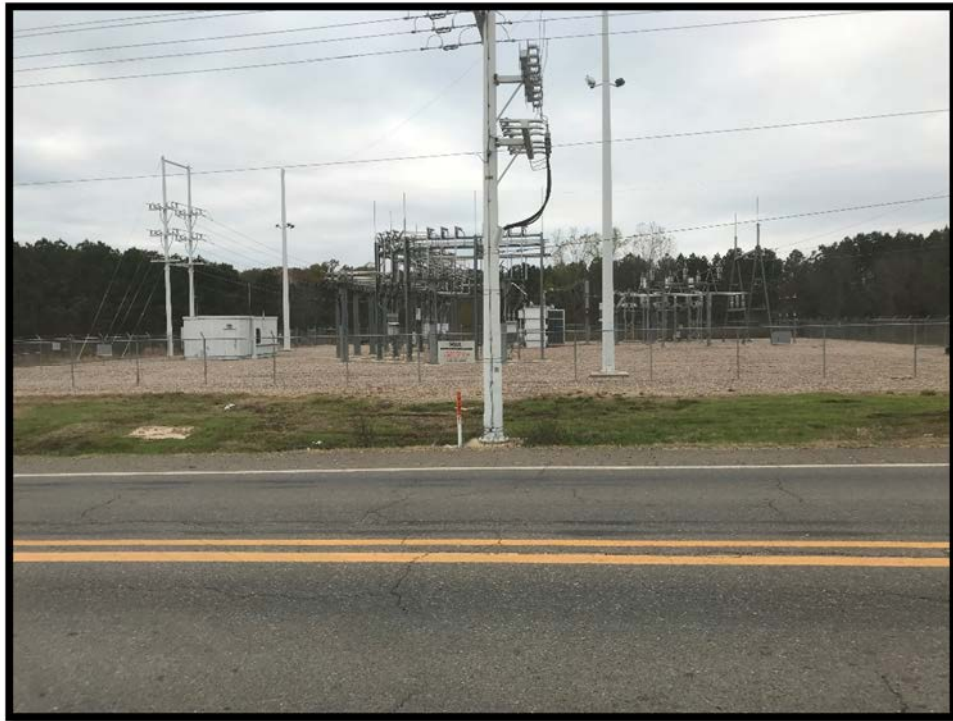
Photo #7 Substation located north of State Highway 32 N.
