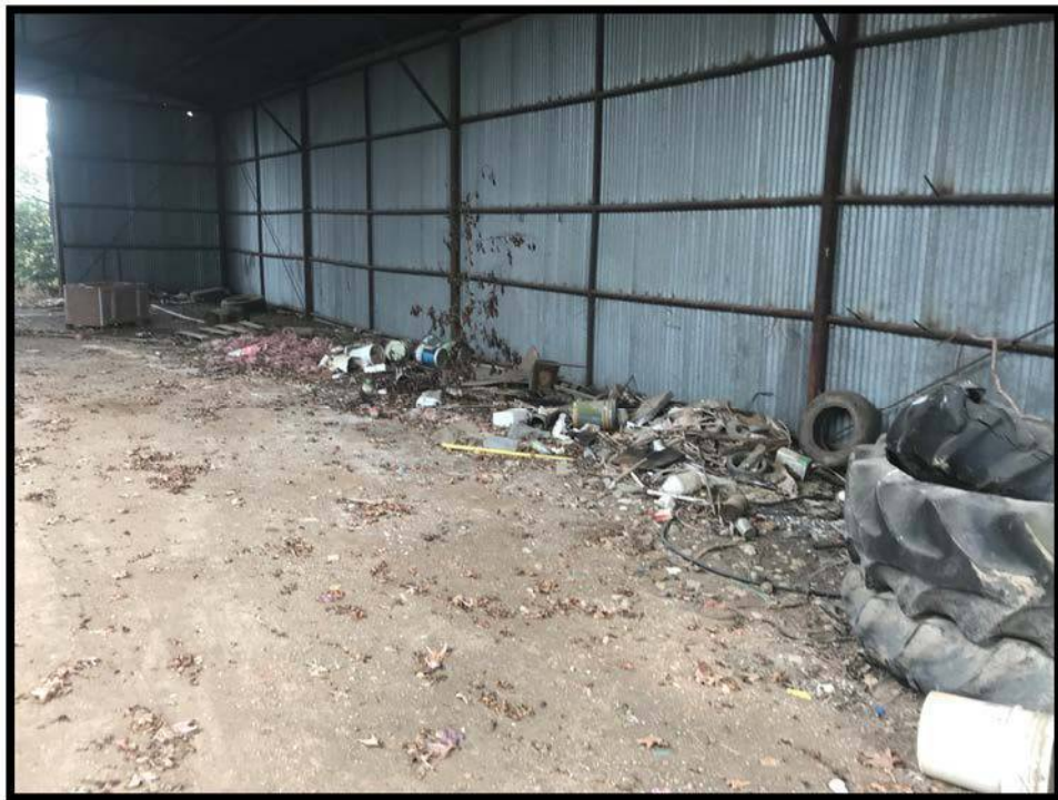
Photo #14 Interior of dilapidated barn located on 162 acre lot.
