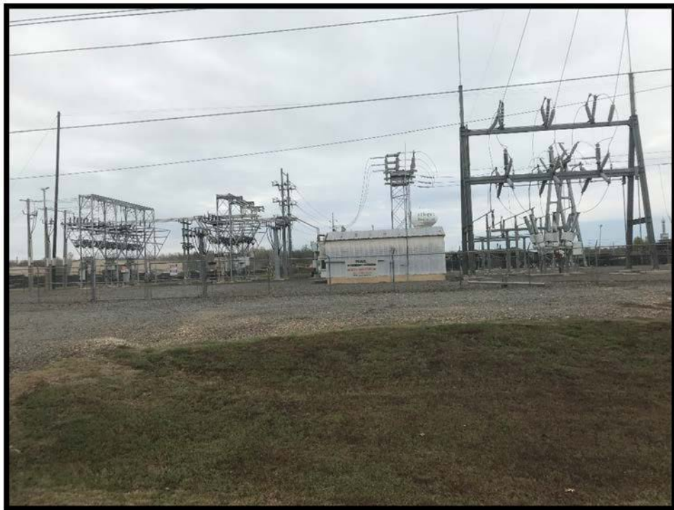
Photo #20 Substation located on eastern side of park.
