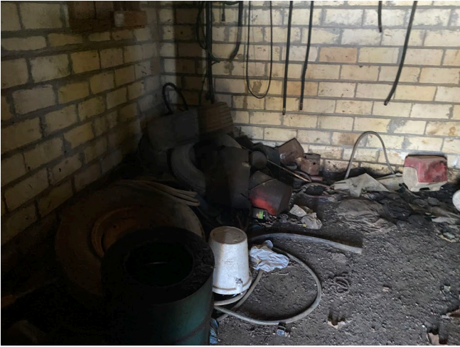
Photo 7: View of former "oil room" in northern adjacent storage building with stained floor and odors.
